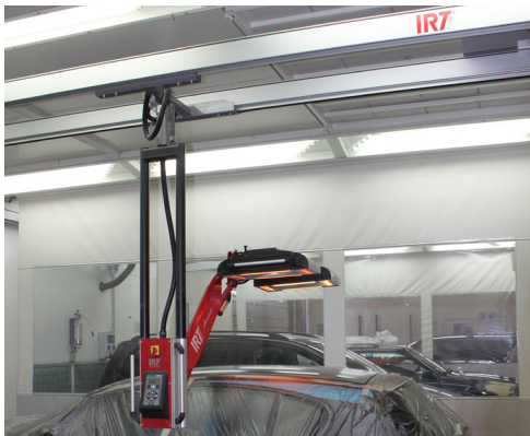
EXAMPLE DRYER IN IRT RAIL
